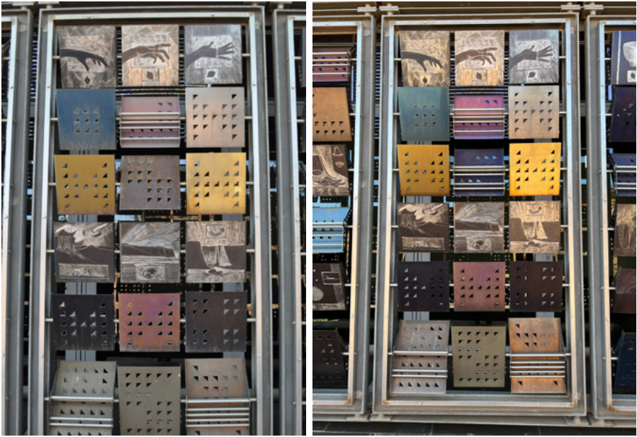
Figure series 31: The sun screens at the Constitutional Court after having been cleaned with dishwashing liquid and water.
